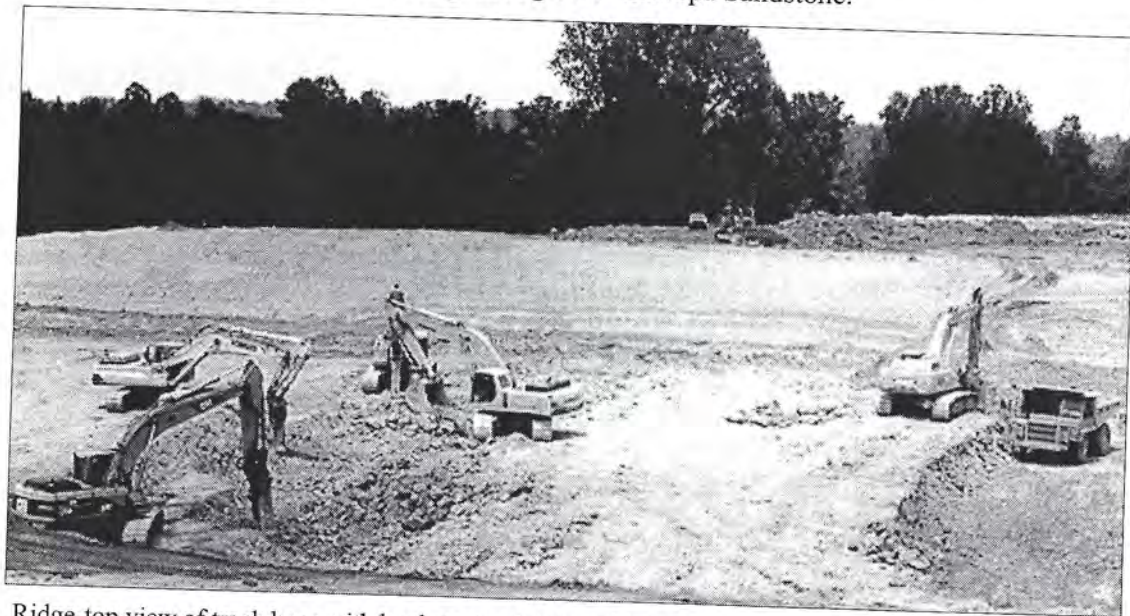
Ridge-top view of track hoes with buckets, track hoes with jackhammers, and a haul truck removing the Chiwapa Sandstone from the Highway 76 cut.
