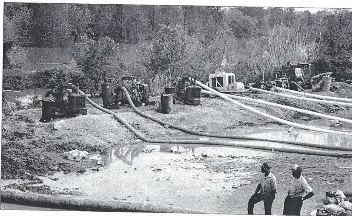
April 17 - Water lines carry flood seepage over a make-shift levee at the Jackson Waterworks.
