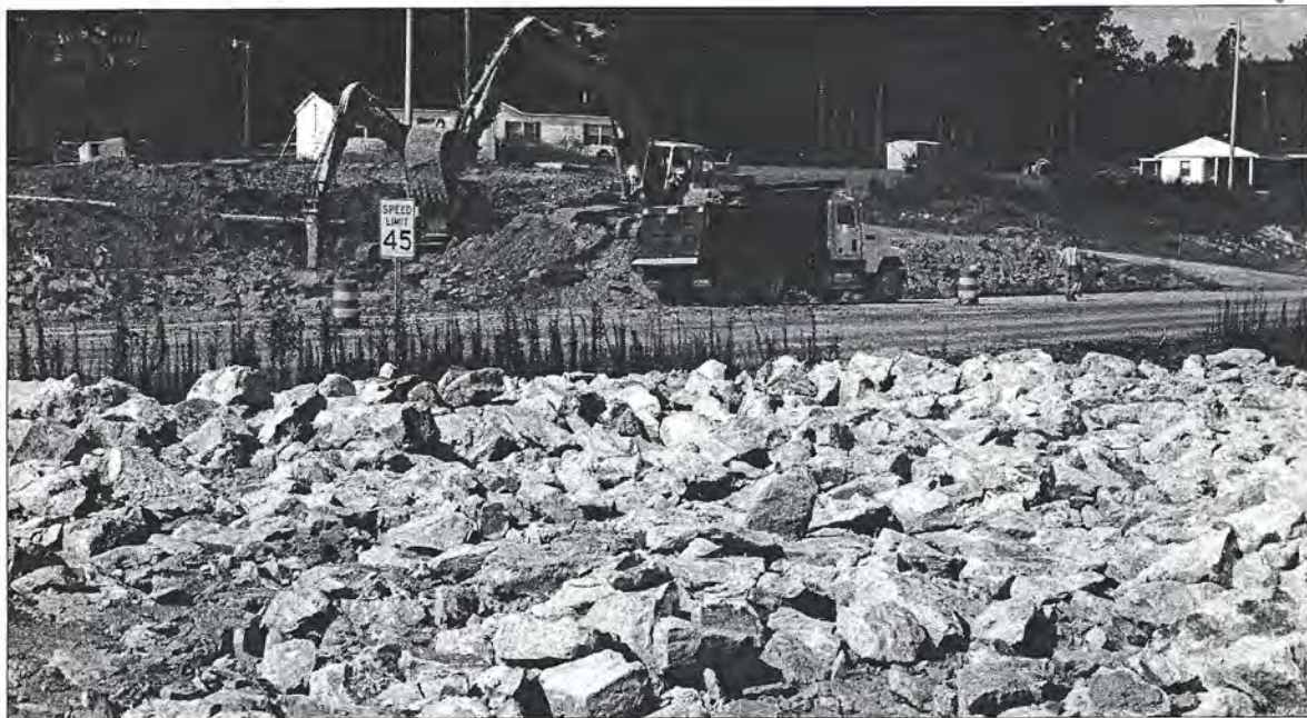
Figure 1 – Jackhammered Tallahatta Sandstone, Highway 16
