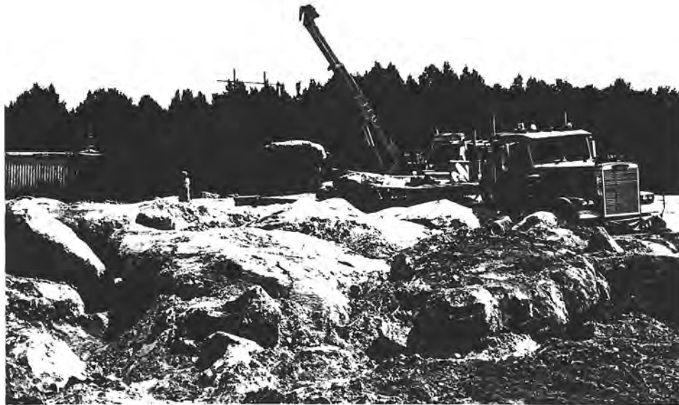
Bashie boulders being loaded on a flatbed truck to be placed in front of the Mississippi Museum of Natural Science
